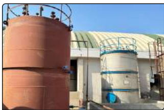
Tank Firm Area
