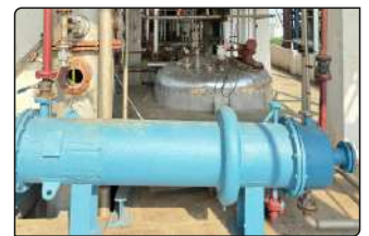
Condenser (Solvent Recovery System)
