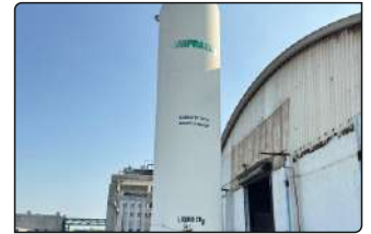
Co2 Tank under PESO ACT.
