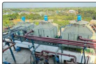
Cooling Tower Area
