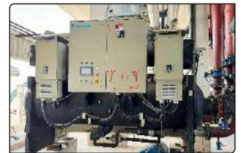
Chilling Plant Area
